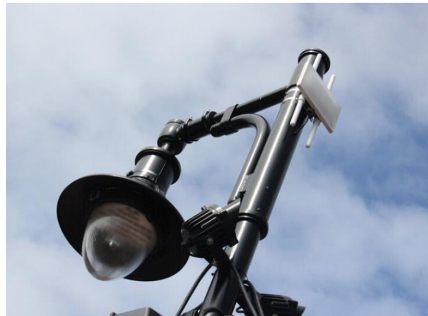
Light pole-mounted Wi-Fi (white box in upper right)
